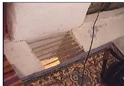
Picture 11. A view of the ventilation opening between the ground floor and the courtyard where the view was taken
